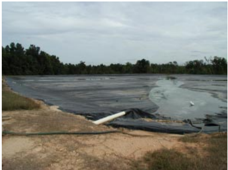
Covered In-Ground Digester
