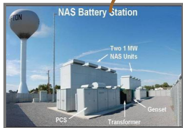
Substation Batteries 10's of MW
